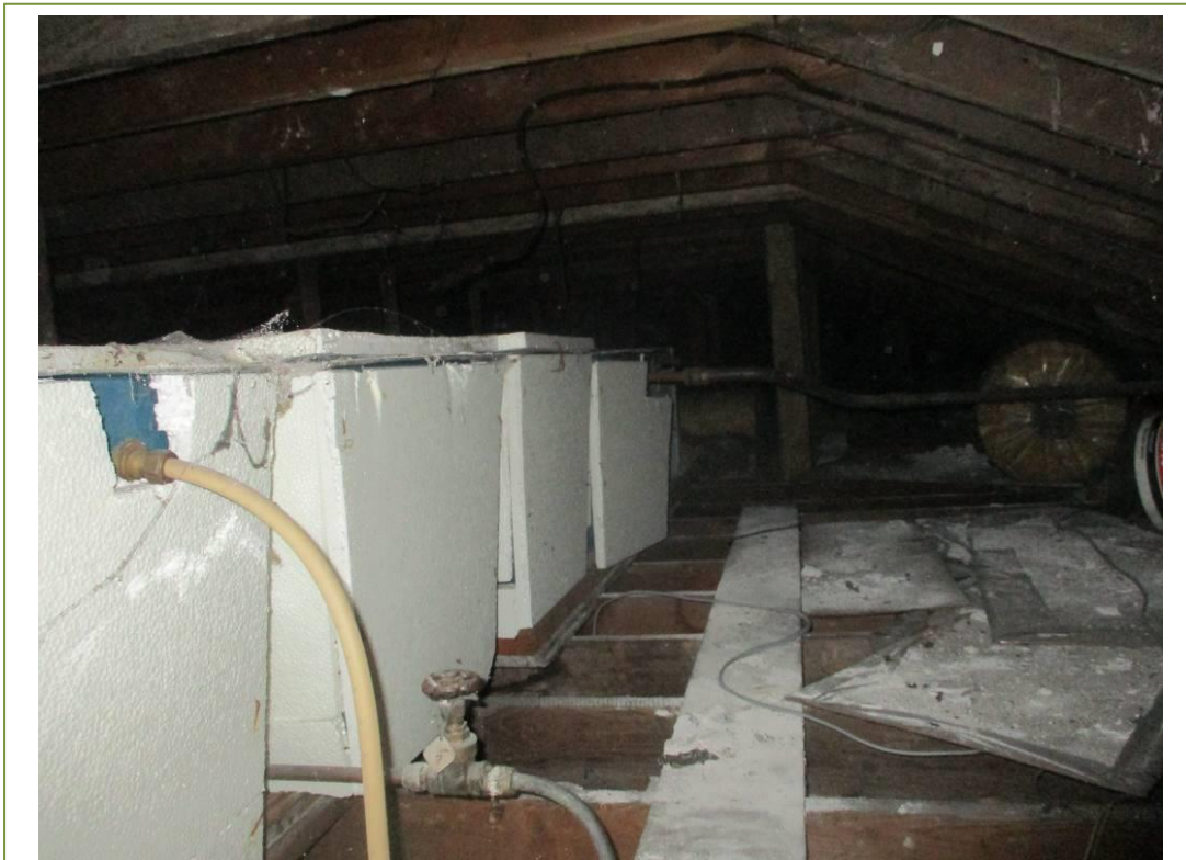
Water tanks in the attic in the main house
