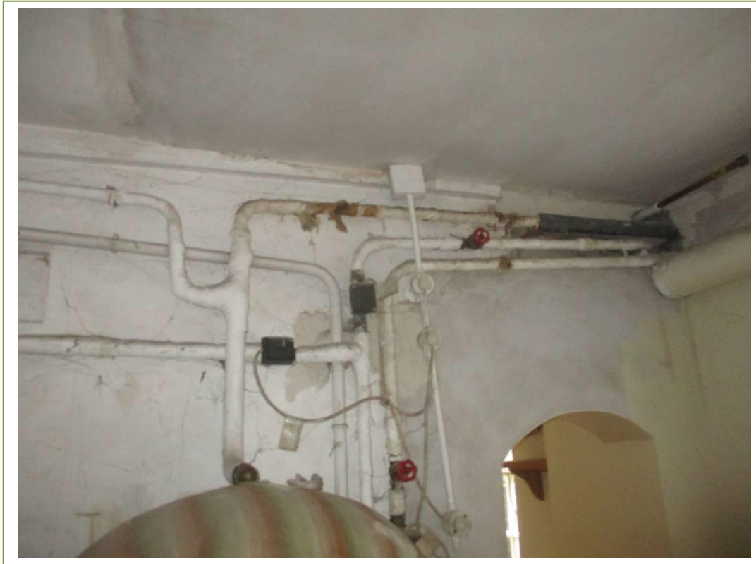
Pipework insulation in the basement kitchen plant room in the main house
