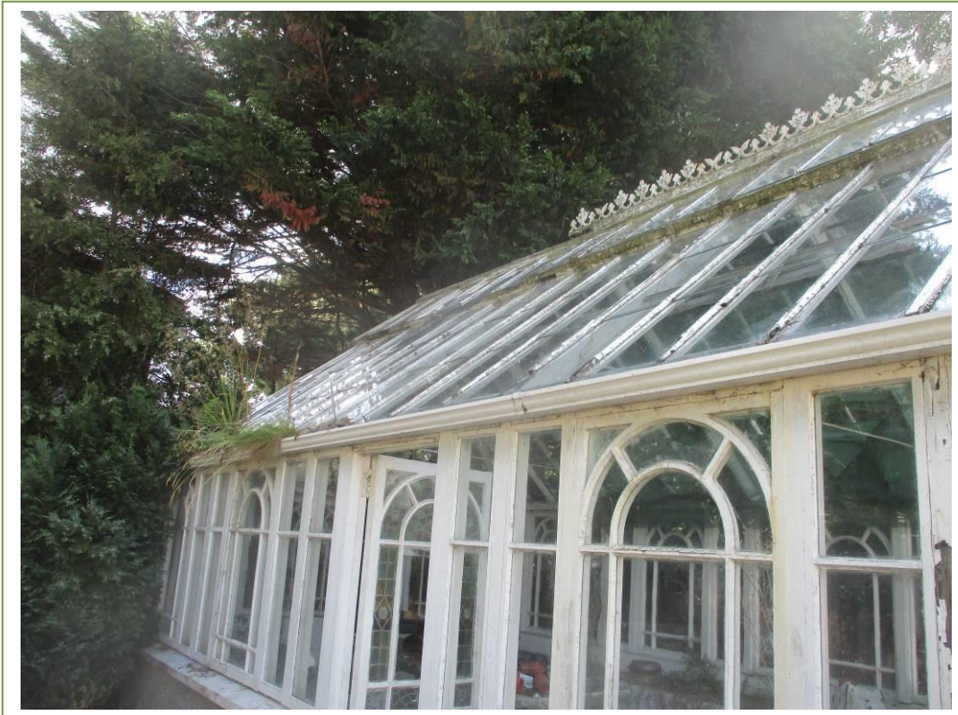
Putty on the glass in the glasshouses
