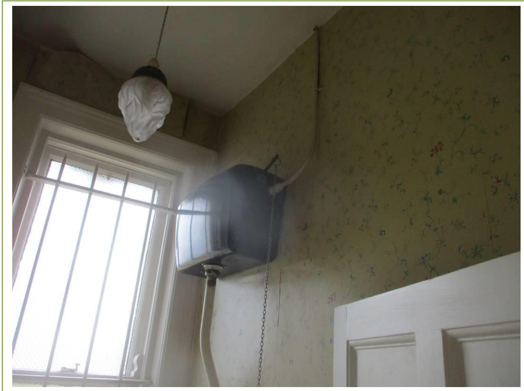
Toilet cistern in the 1 st floor W/C in the servant's wing
