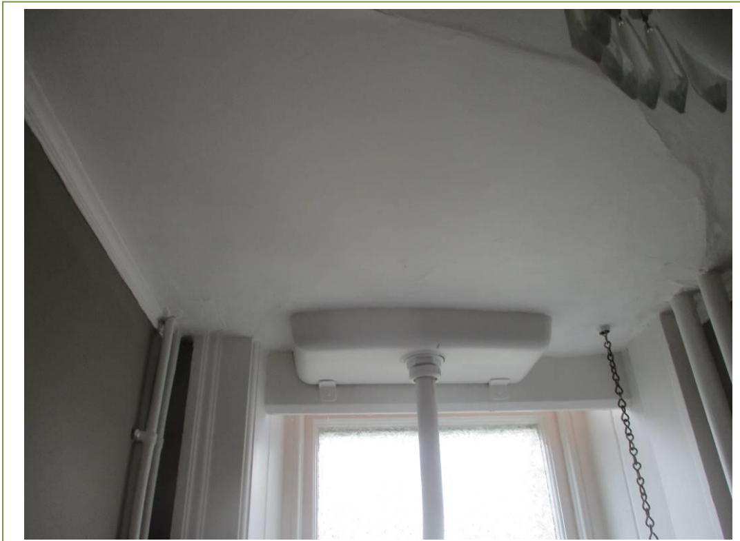
Toilet cistern in the ground floor W/C behind the stairs
